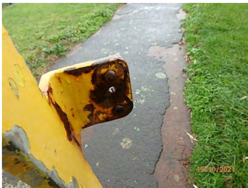
Missing stoppers on gate slam plates
