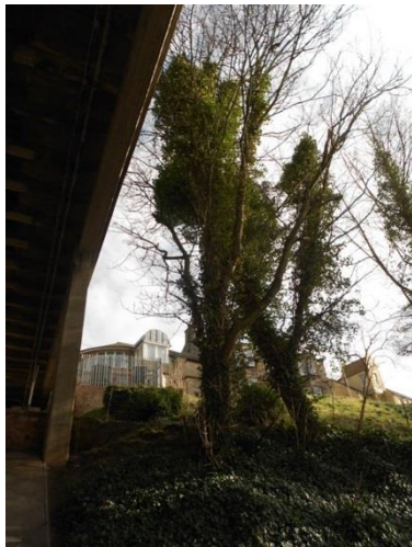
Photo 5 Tree too close to bridge
