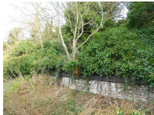
Photo 6 Tree growing on wall top
